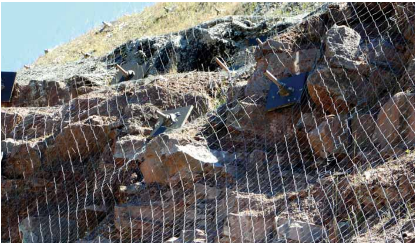
GEWI® Rock Bolts & DELTAX® – Installation at Heads of The Valley Road Improvement Scheme, A465 South Wales
