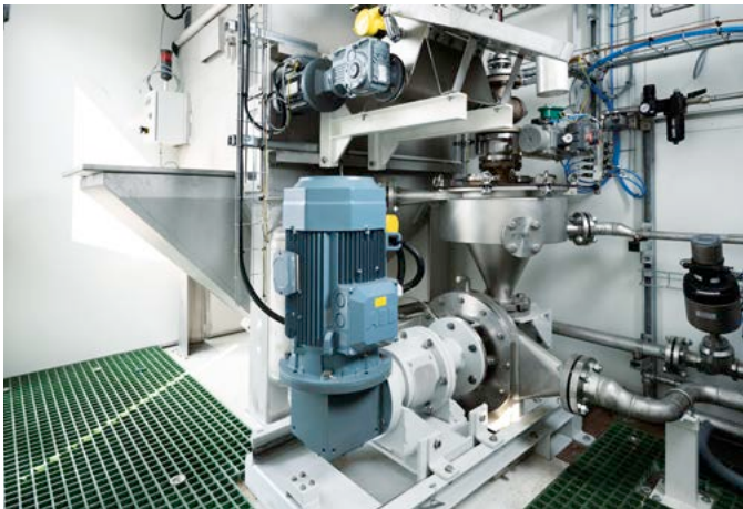
The SIMOTICS CONNECT 400 sensor module mounted on a third-party motor in a plug-and-pump installation from SNF.
