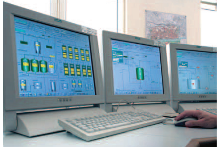
Fig.6: PCS 7 control room
