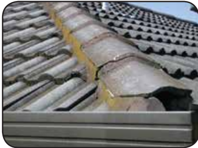
Algae formation on cement mortar
