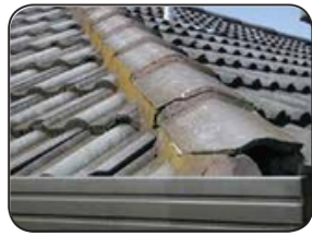
Algae formation on cement mortar
