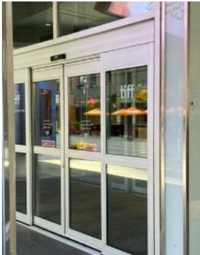
Figure 3: The larger doors on the right side have movement sensors which will automatically open for you.
