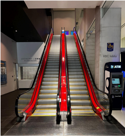
Figure 5: Photograph of the escalators in the front lobby of TIFF Lightbox. The escalator to the right will allow you to move upwards to the second floor.
