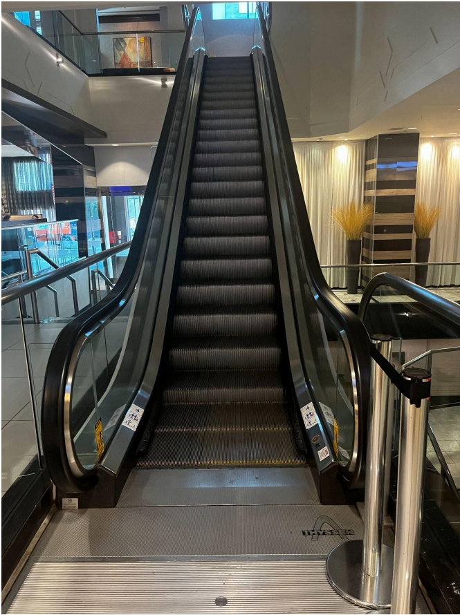
Figure 6: A photograph of escalators.
