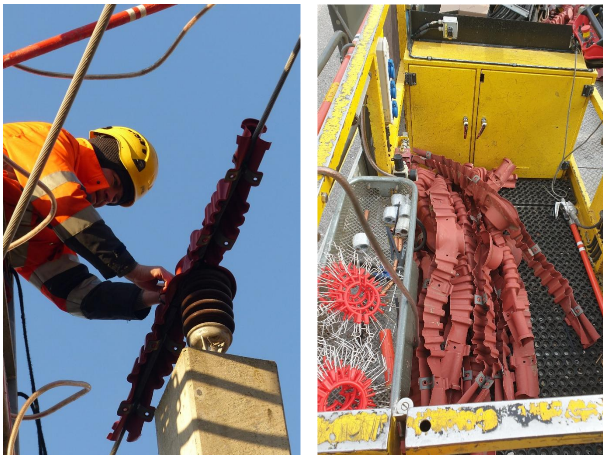
Figure 1: Installation of bird protection devices: a) mounting of protective caps on railway pylon top insulator (Photo: Renate Wunder); b) protective caps (center) and Animal Guards (bottom left) prepared for installation work (photo: ÖBB Infrastruktur GmbH)
