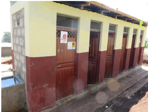
1 PHOTO OF THE SANITATION HARDWARE
