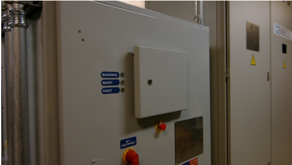
Figure 5-2 Lithium Ion Battery Energy Storage System located at the Black & Veatch Headquarters
