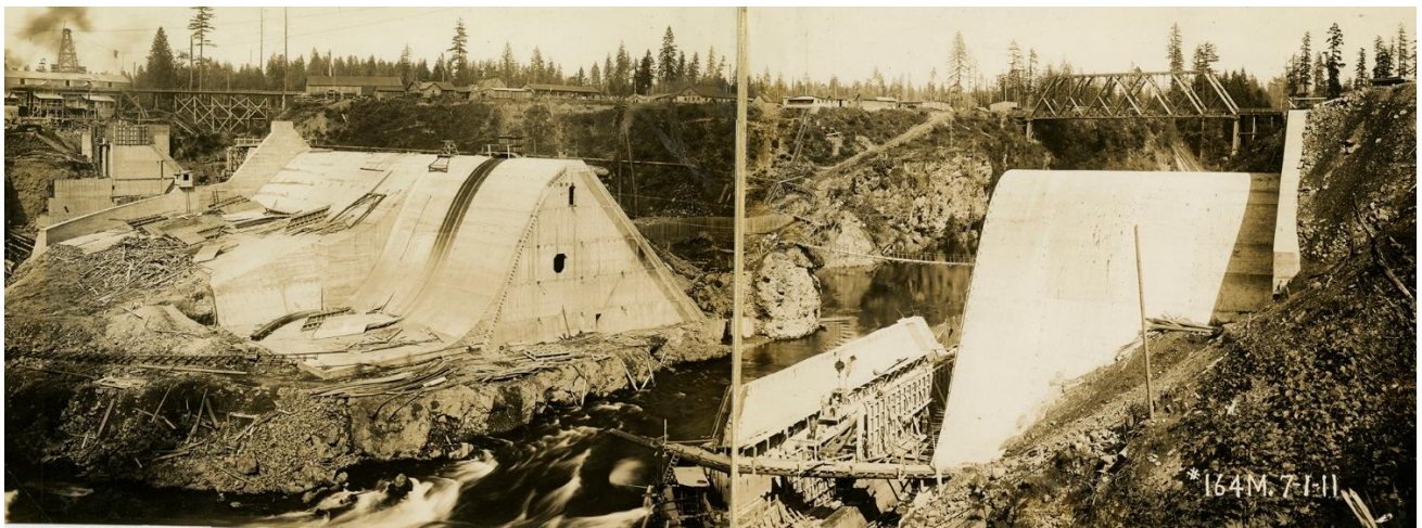
Panorama of the construction of River Mill (originally known as Station M), taken on Oct. 28, 1911.
