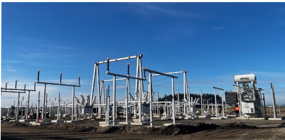
Newly updated Monitor Substation
