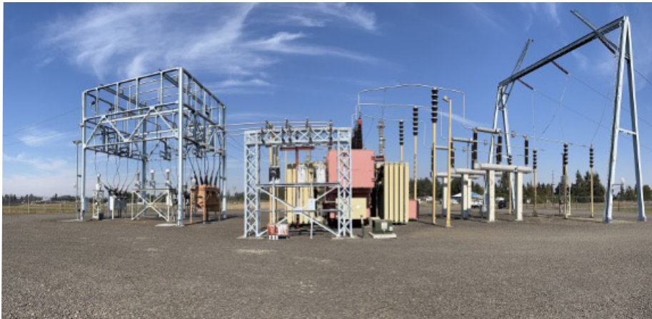
Old equipment at the Monitor Substation
