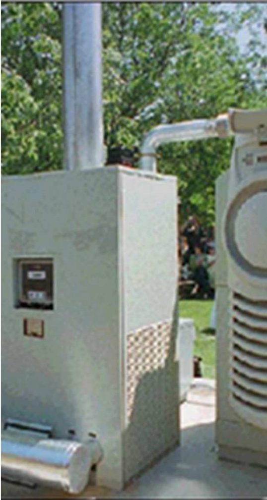
Microturbine with Heat Recovery
