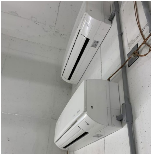
Figure 26. Mounted Cooling Heads
