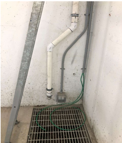
Figure 33. Drain Line and Sump Grate
