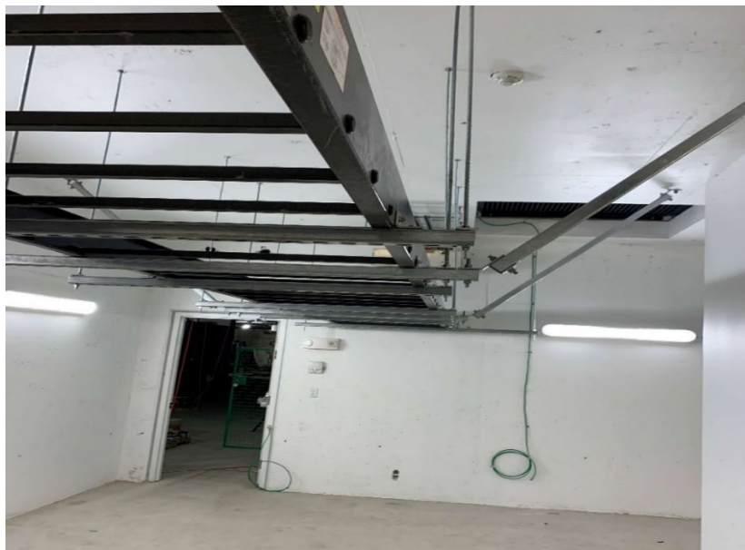
Figure 32. Secondary Cable Tray
