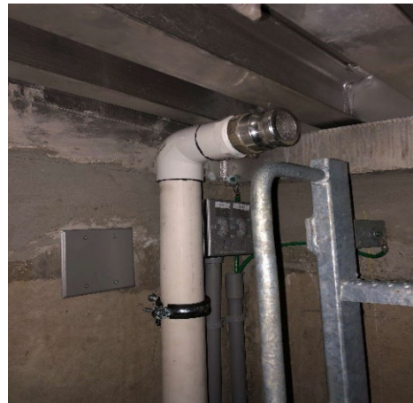
Figure 34. Drain Line at Door
