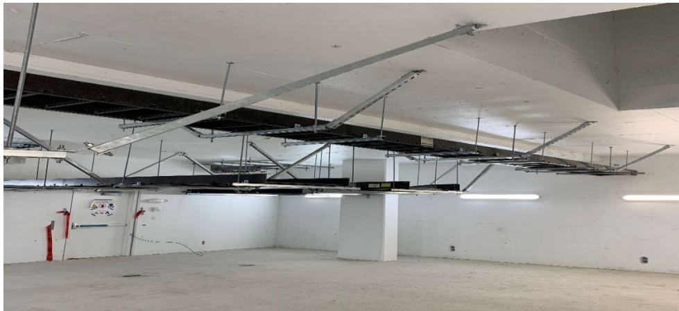
Figure 31. Primary Cable Tray
