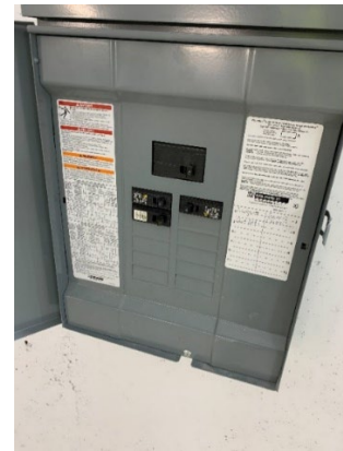
Figure 25. NEMA 3 Breaker Panel
