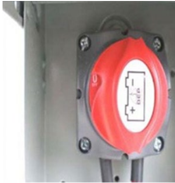
Figure 11. DC Switch Inside a Disconnect Panel
