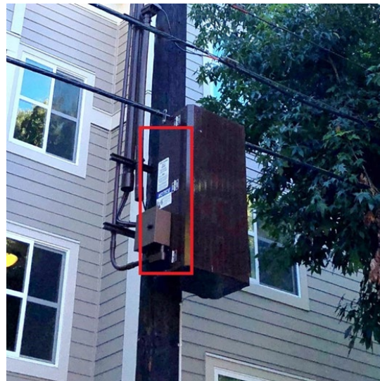
Figure 14. NOC Information and RF Safety Signs on Wireless Equipment Cabinet
