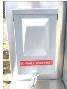
Figure 10. Close-Up of DC Disconnect
