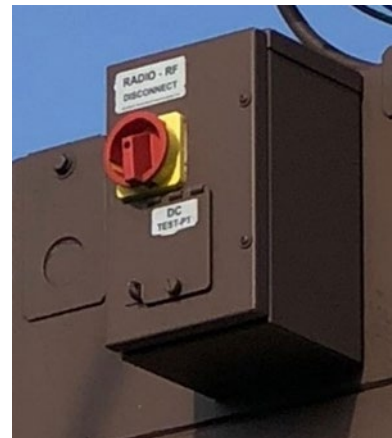
Figure 13. Close-Up of AC Disconnect Switch
