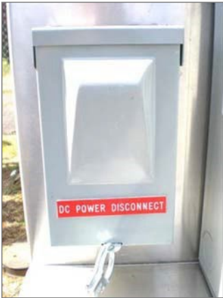
Figure 8: Close-Up of DC Disconnect
