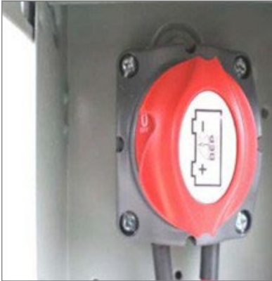
Figure 9: DC Switch Inside a Disconnect Panel
