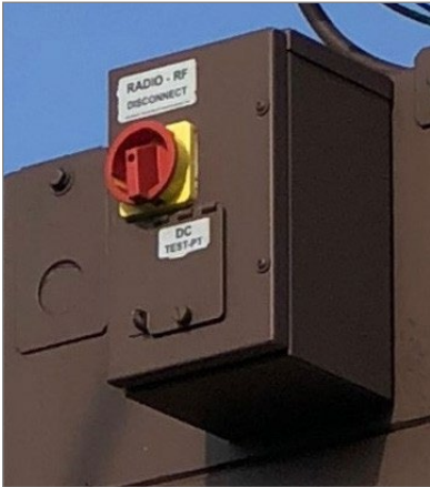
Figure 11: Close-Up of AC Disconnect Switch
