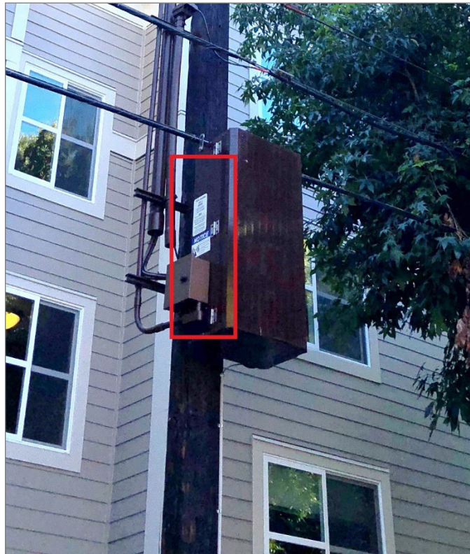
Figure 12: NOC Information and RF Safety Signs on Wireless Equipment Cabinet
