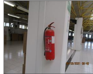
Photo of fire safety equipment Fire extinguisher.JPG
