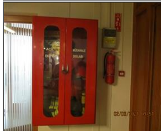
Photo of fire safety equipment Firefight equipment.JPG
