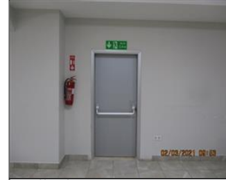
Photo of fire safety equipment Emergency exit.JPG
