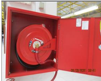
Photo of fire safety equipment Fire hose.JPG
