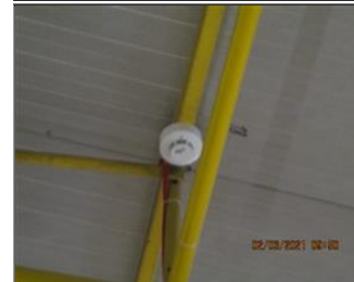
Photo of fire safety equipment Smoke detector.JPG
