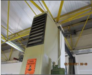
Photo of the inside of the main production hall Heating system.JPG
