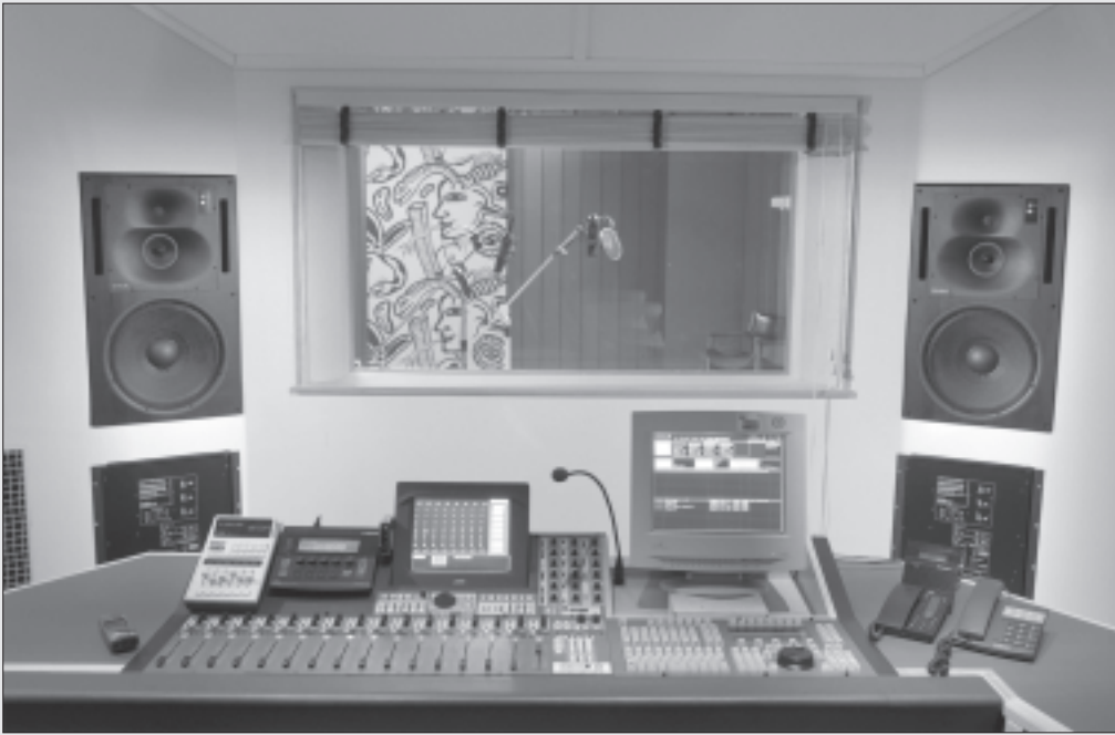
Stockholm City Theater Control room 1
