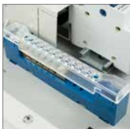
Neutral Bars [covered]
