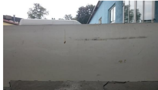
TE Adhesive Failure
