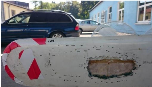
Simulated lightning damage
