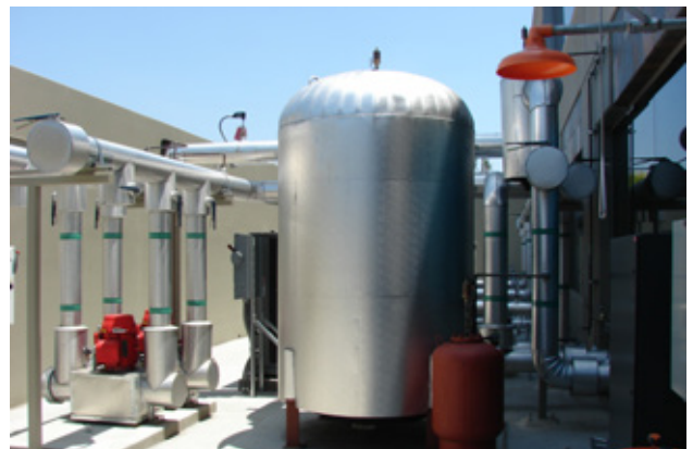
We have invested in an energy efficient cooling system for our lab in Calabasas, California.
