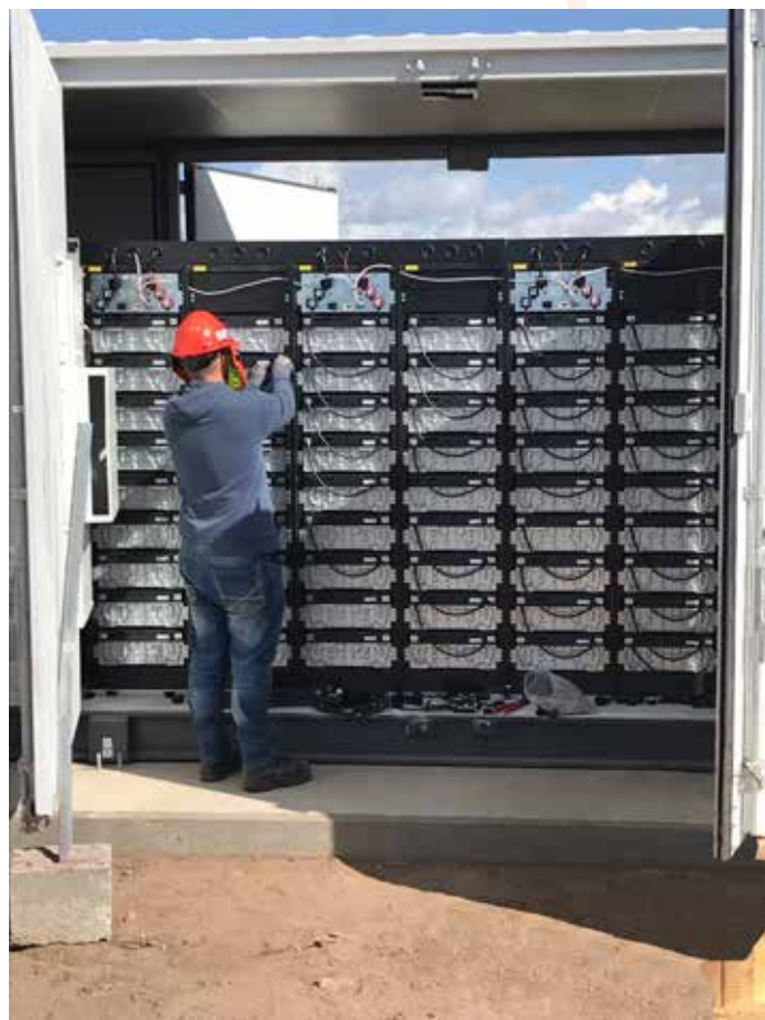
Battery energy storage system at Panguitch's 650 kWac monocrystalline photovoltaic (PV) plant.
