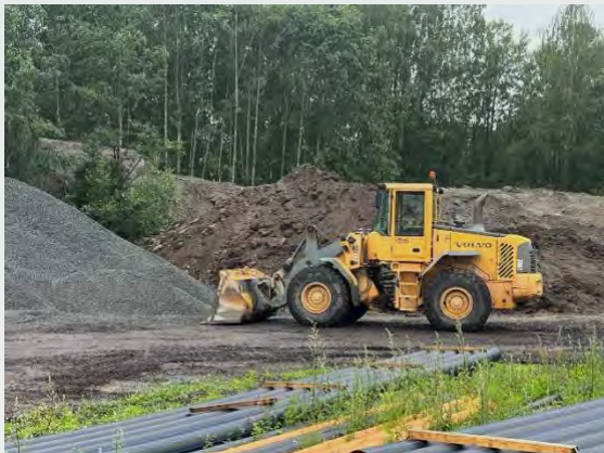
The plot at Follum was prepared for groundwork during the second quarter.
