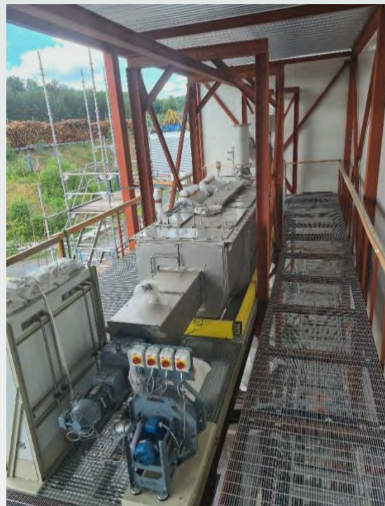
Process equipment, including the pyrolysis reactors installed.
