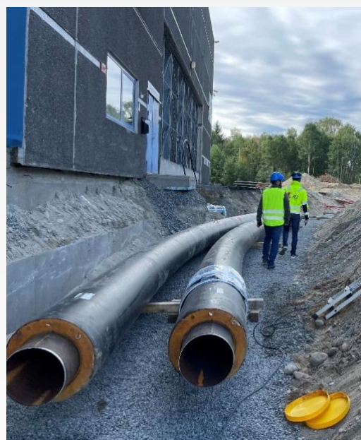
Infrastructure was completed in December 2023, connecting the local district heating company, Vardar Varme to the production plant.
