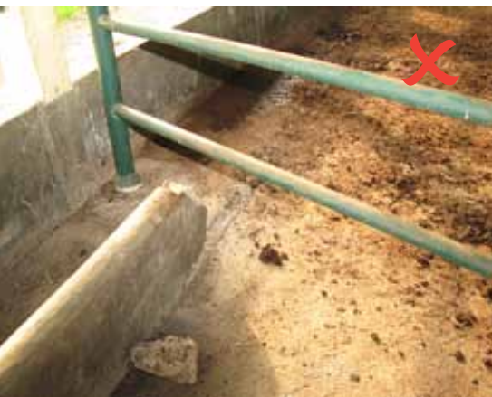
Repair all damage to feedlot facilities.
