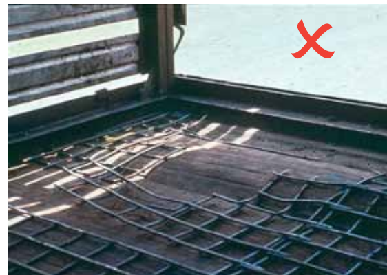
Steel mesh for reinforcing concrete is too light and needs to be replaced if it breaks up.
