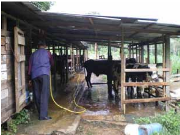
The low height and shallow pitch of this roof would make the shed very hot in summer and contribute to heat stress.
