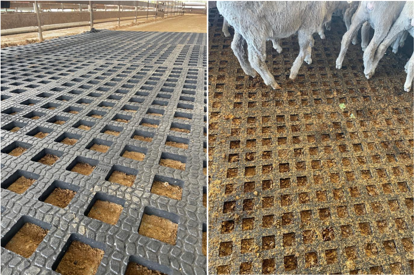
Images: Installation of the Kura mat, the top preference by facility staff.
