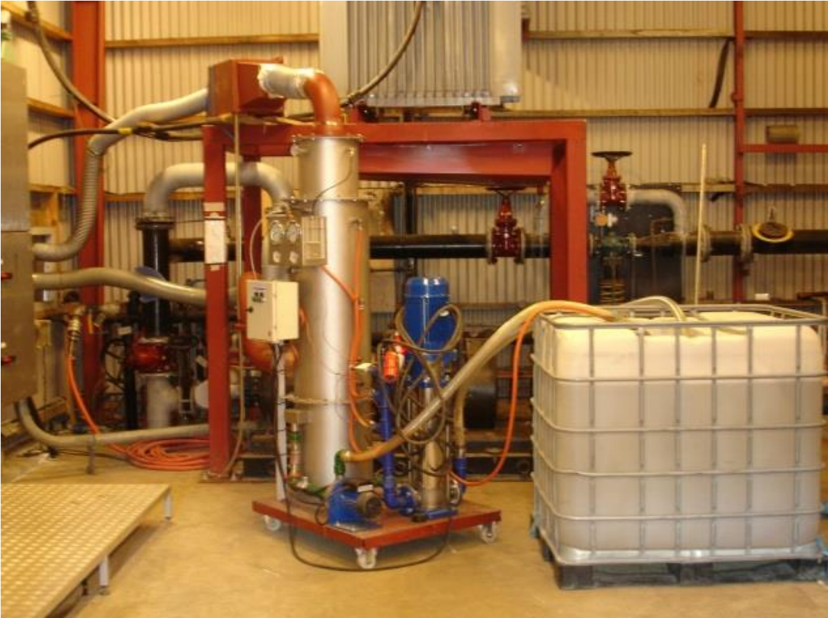
Our Exhaust Gas Cleaning Facilities
