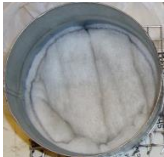
Soot in a filter (system with scrubbing equipment)
