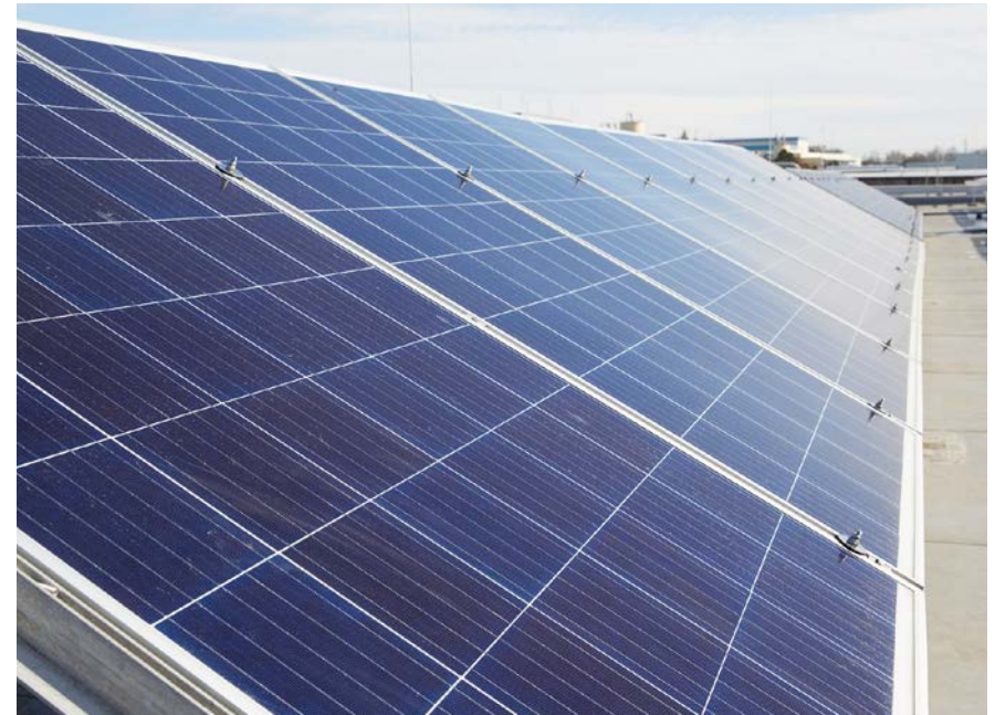
Own photovoltaics power generation: Our PV systems generate enough energy to cover the annual electricity consumption of 160 single-family homes.
