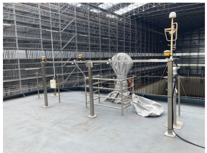
Figure 3: A-2-Sea designed an antenna mounting frame to provide an optimal location for GNSS data reception.
