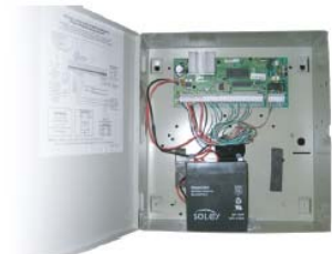
Backup Power Supply
