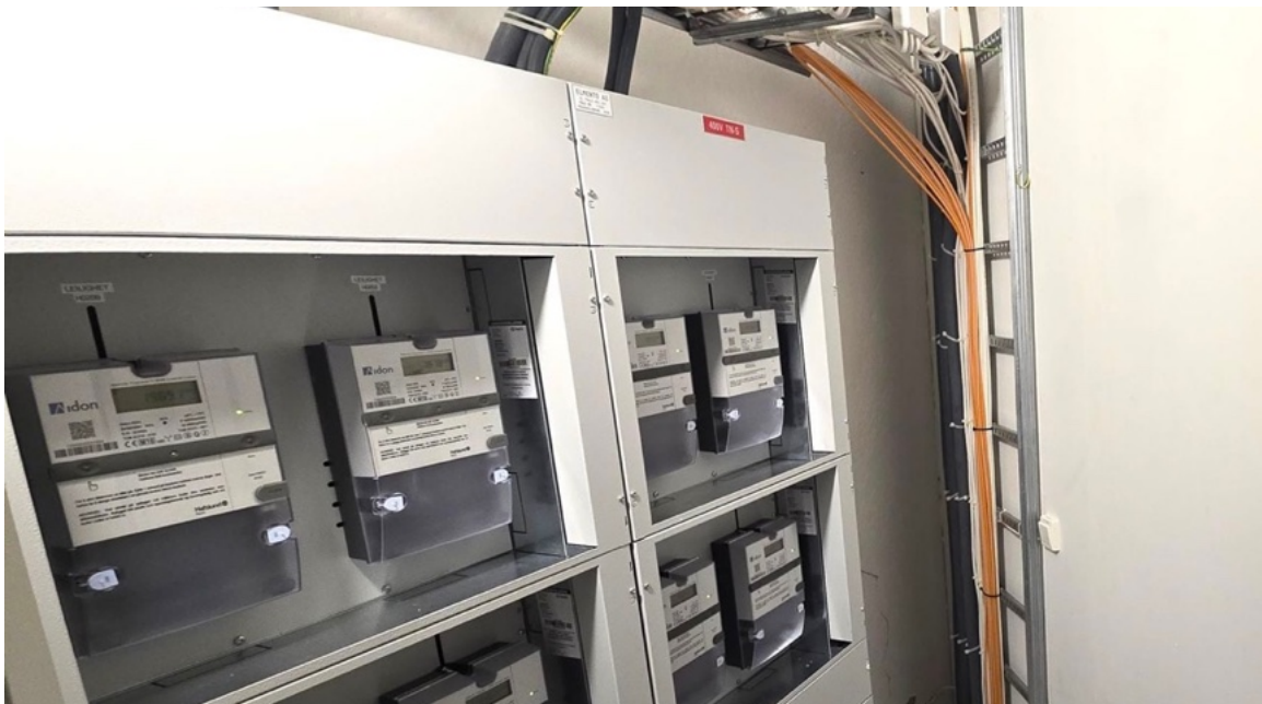
Picture: Electrical equipment at pilot site, Norway 2026
