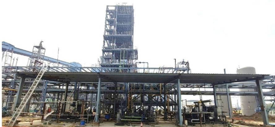
Fig. 3. Photograph of the 10 TPD Methanol synthesis pilot plant installed at NTPC Vinhyachal.
