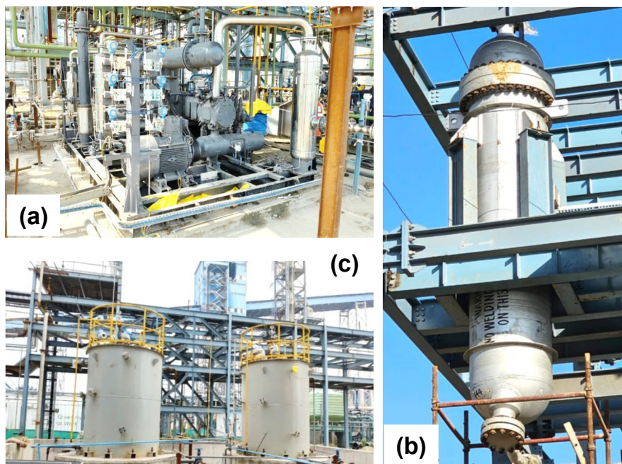
Fig. 5. Photographs of the key equipment installed in the pilot plant. (a) CO 2 Compressor, (b) Methanol Reactor, and (c) Product Methanol Storage Tanks
