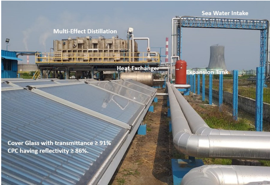
Fig. 3. Single collector ETC-CPC, with Toughened Glass Cover and Multi Effect Distillation over the structure.
