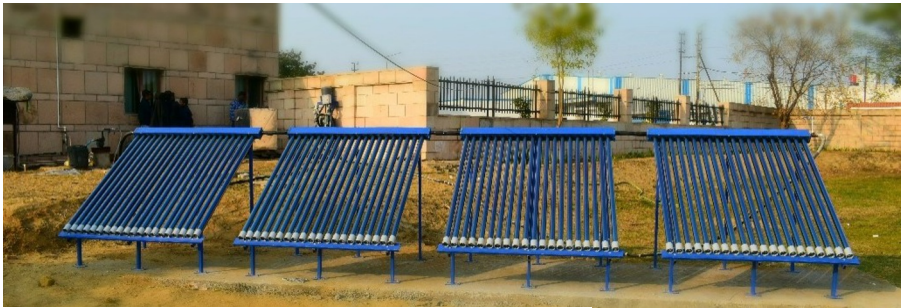
Fig. 5. Photograph of the Installed system.
