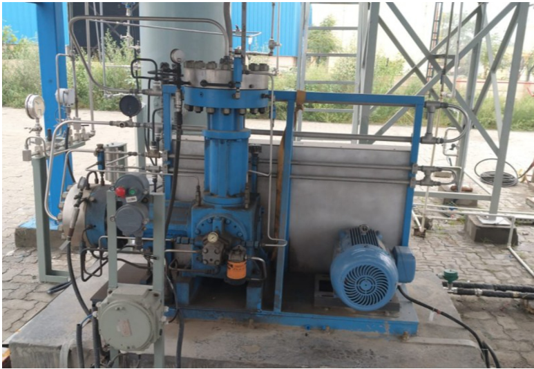
Fig. 8. Site photograph of the Diaphragm Compressor
