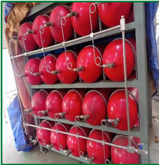
Fig. 9. Site photograph of the Hydrogen Storage.
