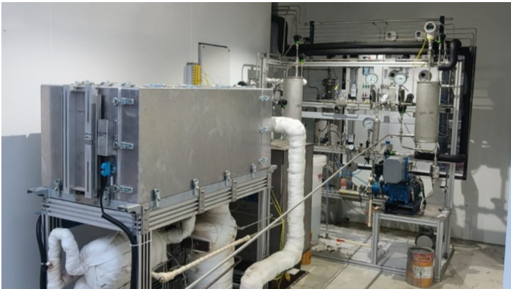
Fig. 6. Site photograph of the TSE System showing various components.
