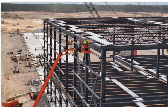
The first steel beams went vertical on the Scout Motors construction site in May.
