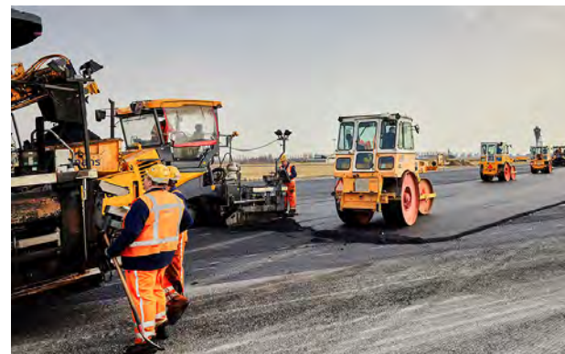
60% of the original asphalt from the Polderbaan Runway was reused as it underwent maintenance.
