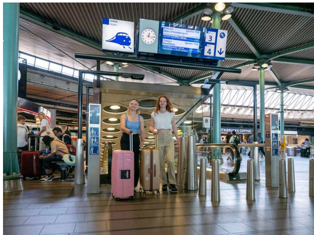
At Schiphol Plaza the project has started to enhance the capacity to and from the platforms by renewing staircases and elevators.
