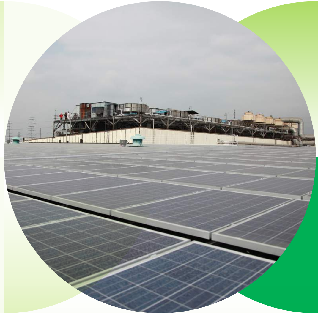
Our Huangpu plant in China partnered with a local utility supplier to install solar panels on the plant's rooftop. This is the first P&G manufacturing plant in Asia to host solar PV panels. Electricity from the installation will eliminate 600 metric tons of CO 2 emissions annually from the local community.
