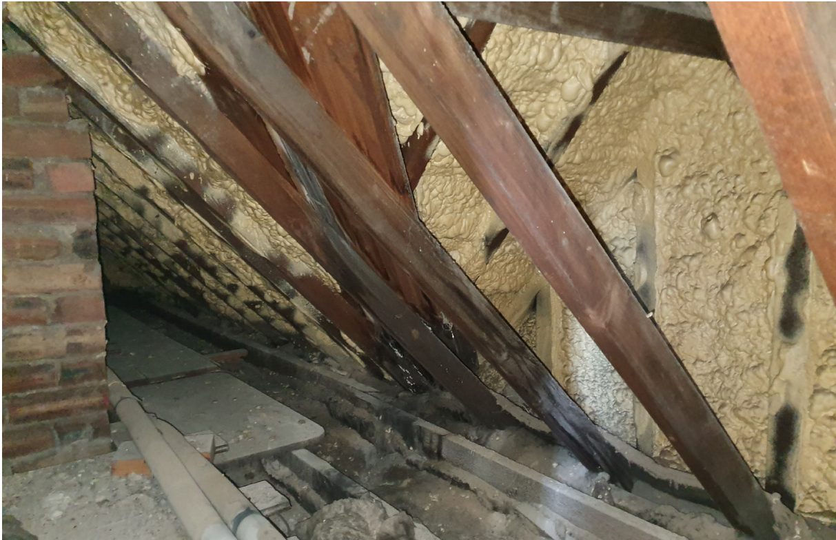
Figure 4: Example of spray foam incorrectly installed leading to condensation problems
