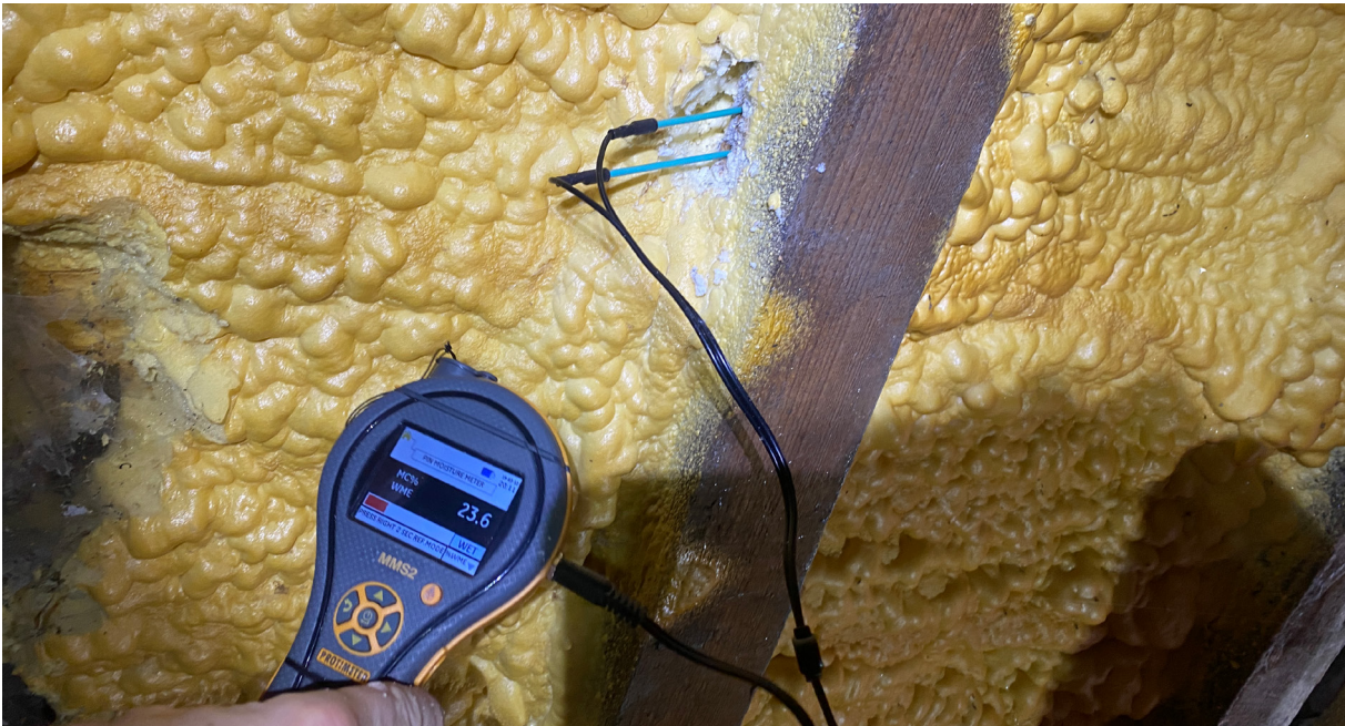
Figure 3: Spray foam insulation can make it difficult to identify problems to the roof because the timbers can be 'dry' on their exposed, visible surface but 'wet' behind the spray foam
