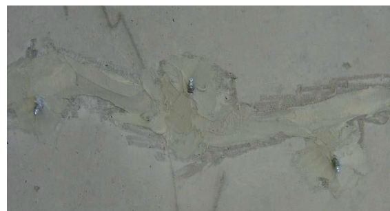
Figure 1. Socket type nipples placed around the crack and sealed with proper epoxy adhesive from MasterStrength® series.
