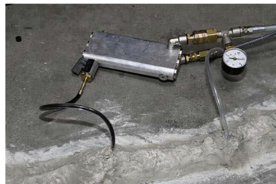
Figure 3. Injecting MasterFill® ER I380 by using a 2C pump to repair a concrete floor.
