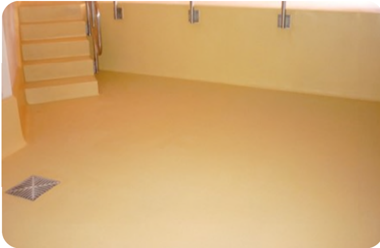
Ucrete DP floor in the Tanker Reception Bay
