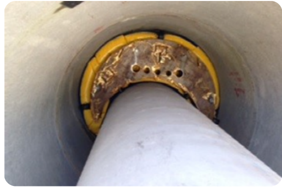
Mock-up of the inflatable bags after filling with precision grout sealing the tunnel annulus
