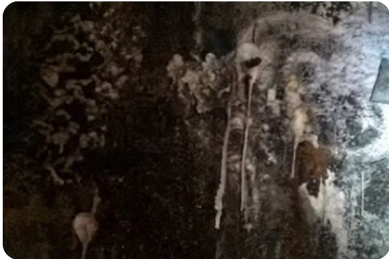
Weeping shotcrete without the MasterLife 300D
