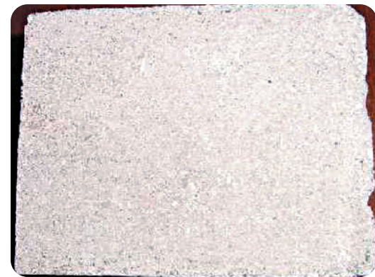
Figure 10: Portion of a concrete paver with a homogeneous thick film of calcium carbonate efflorescence resulting from water condensation and subsequent evaporation.
