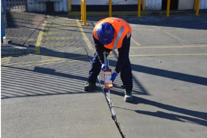
Joint sealant is applied to the cleaned joint after backer rod application
