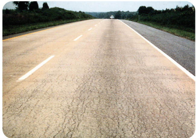
Figure 1. ASR-Induced Map Cracking in Pavement
